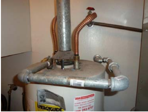
Drain line contrivance. Not permitted!
