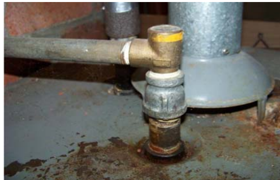
Wrong safety valve not permitted.
