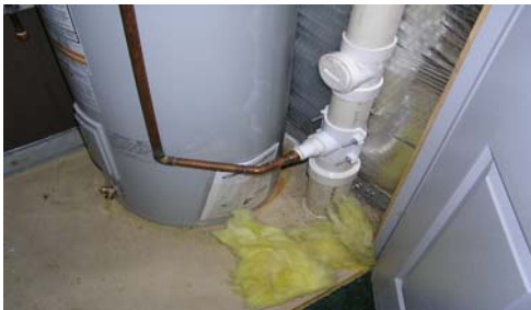
Direct to sewer not permitted.
